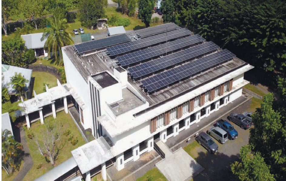
The Pacific Climate Change Centre in Apia is fully powered by the sun, with 20% of the solar panels on its roof funded by Japan. PCCC
